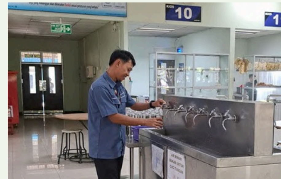
► Fasilitas sarana RO yang berada di Kantin 1 Perseroan. | Reverse Osmosis (RO) facility located at the Company's Canteen 1.
